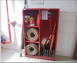
Photo of fire safety equipment Fire fighting equipments.JPG
